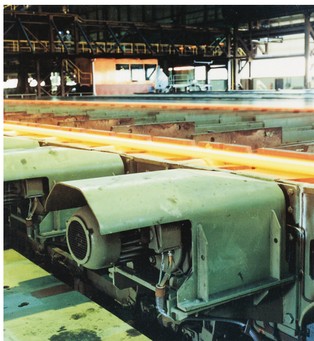
Fig. 4.8.1.6 Roller table drives on a cooling bank protected by a cover against mechanical damage caused by the red-hot material being conveyed
