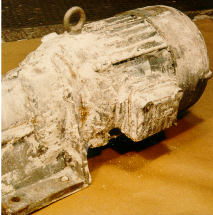
Fig. 5.4.2.3 Fouled cooling ribs increase the degree of heating
