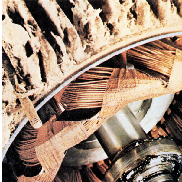
Fig. 3.2.2.4 Severe impairment of cooling on a surface-ventilated motor due to partial blockage of the cooling fins
