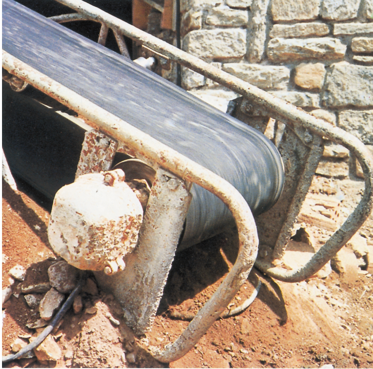
Fig. 4.7.3 Drum motor on a portable belt conveyor operating in arduous conditions on a construction site
