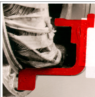
Bild 4.5.4.1 Crowding between the end winding and bearing bracket give rise to flashovers in the presence of condensation. A drain hole would not help in these circumstances.
