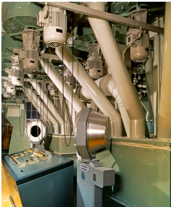
Fig. 10.10.7 Example of the high demands placed a geared motor's seal Shaft aligned vertically up (V3) on cellular wheel sluices in a mill
